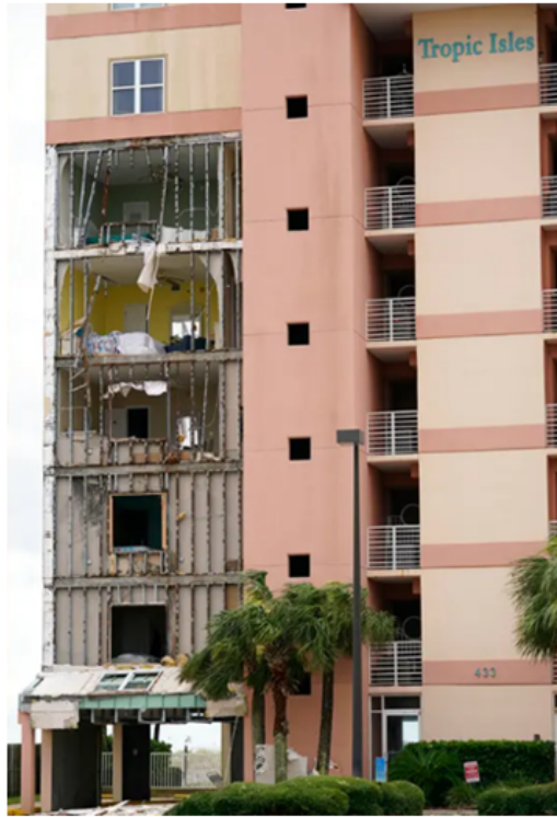
Figure 5: Tropic Isles condominiums are seen after Hurricane Sally moved through the area, Sept.16, in Orange Beach, Alabama Image courtesy of Gerald Herbert Alabama
