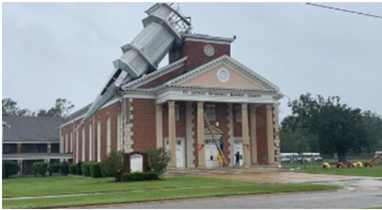
Figure 4: Fallen steeple at El Primitive Baptist Church, Mobile, Alabama Image courtesy of Armondo Moralez (Alabama church steeple toppled as Sally tears through Mobile | Fox News) https://www.foxnews.com/us/alabama-church-steeple-toppled-sally-mobile
