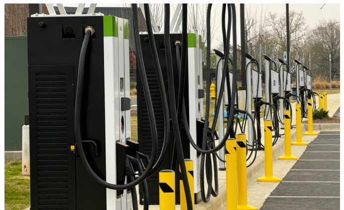
The Montgomery County Commission received an electric vehicle charging grant to install these chargers at Montgomery Whitewater, which attracts paddlers throughout the United States.
