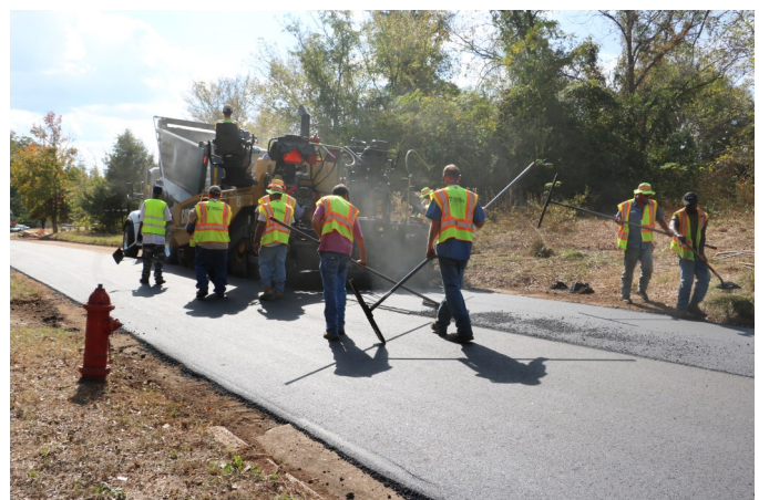
Community Development Block Grants help many Alabama cities and counties with road improvements.
